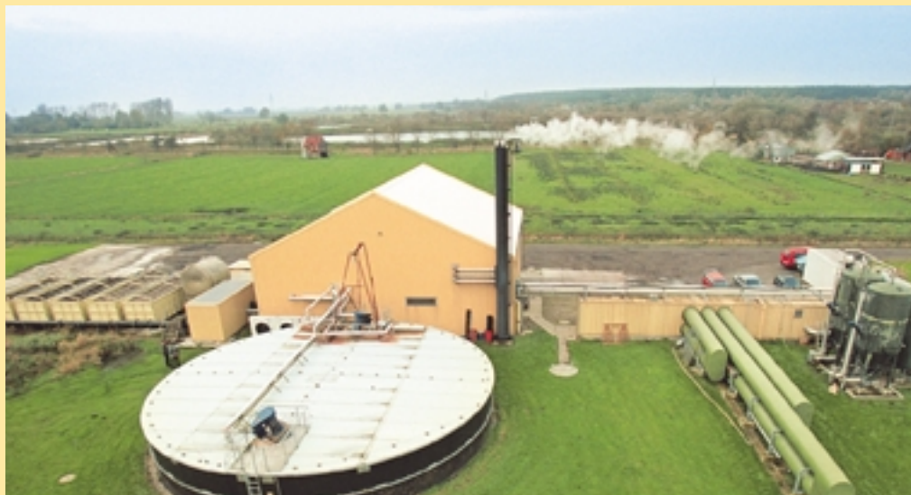
Biogas plant in Schleswig-Holstein, Germany
